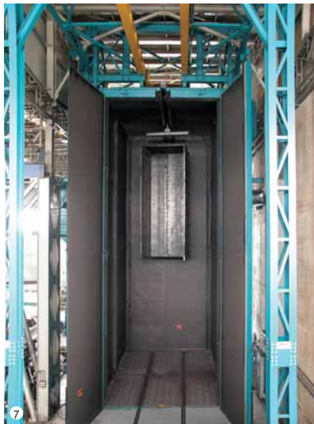
Figure 7: The inside of the shotblasting chamber.
